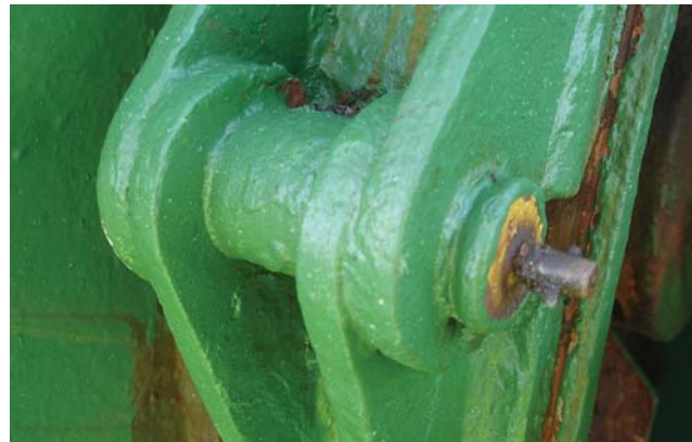
Ineffective grease point
