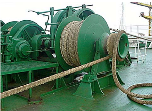
Well painted but poorly highlighted mooring station
